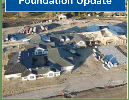
An overhead photo of the new Story Medical Senior Care under construction adjacent to the medical center.
